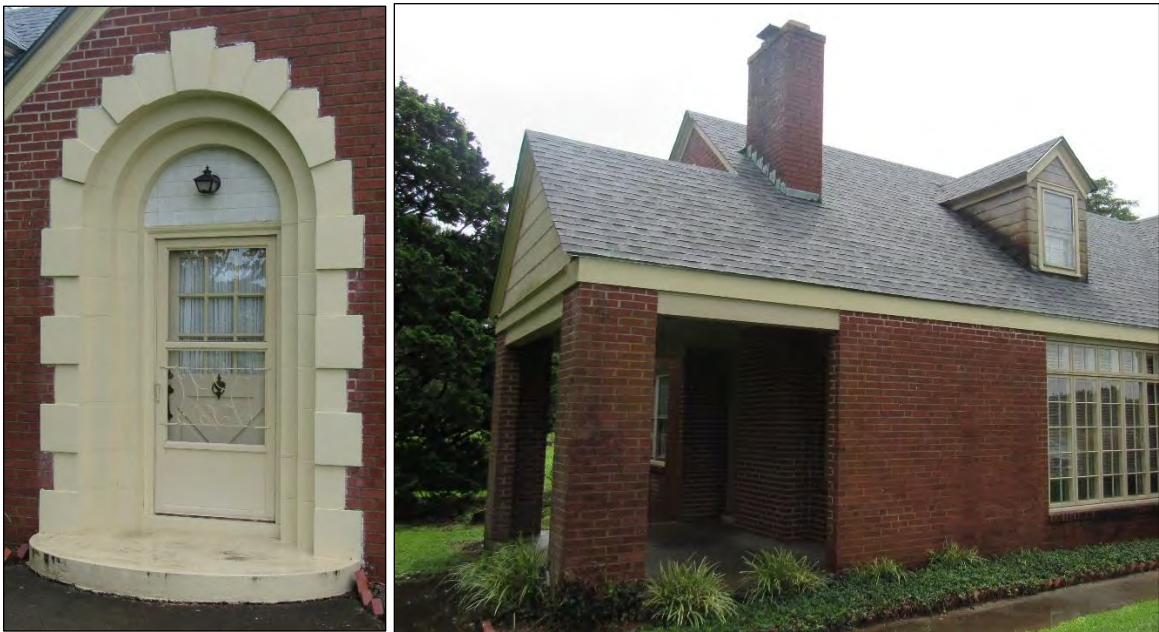
Photo 3: Detail of Primary Entrance (Left); Detail of Side Porch, Northwest Oblique (Right).
